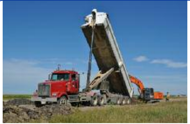
Stewart Hurrell dumping material for Devon Belley to repair a soft spot with John Klassen overseeing things. Picture by Rick Beck
